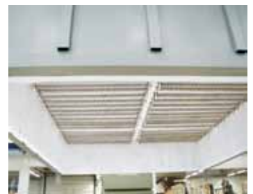
Heating elements in furnace hood
